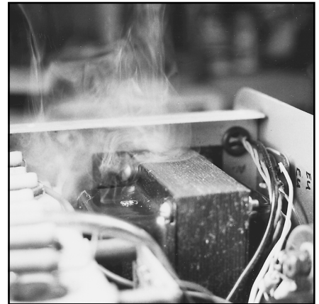
Figure 4—After loss of smoke, the transformer was inoperative.
