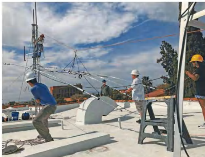
K7UAZ club members raising the new Mosley TA-63N antenna on the roof of the university's Old Engineering building, using an intricate system of pulleys and a tram line. [University of Arizona Amateur Radio Club, K7UAZ, photo]
