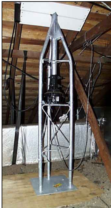
Figure 1—A top section of Rohn 25AG2 nestles comfortably in the attic. V-notched boards fastened to the roof rafters clamp the neck of the tower sleeve. A mating base plate secures the bottom end of the tower section to the ceiling joists below.
