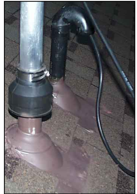
Figure 4—A two-inch to three-inch rubber flexible drain connector keeps water from running down the two-inch-OD mast and between the mast and the tower sleeve.
