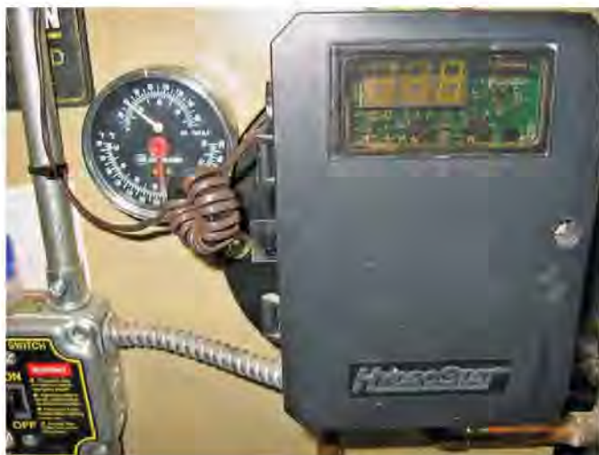
Figure 3 — Winding about 14 turns of the thermostat line through a Type-43 ferrite core kept RF out of this oil burner control. [Dan Bowman, K1FEV, photo]
