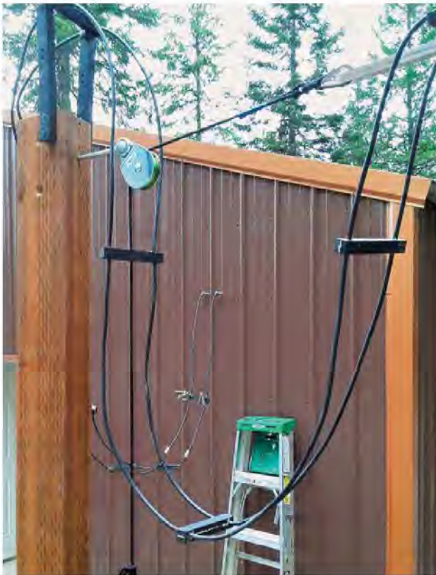
The rope runs through a pulley and is then tensioned with a counterweight seen against the post in the foreground. Half-inch electrical conduit comprises the shack wall feed-throughs.
