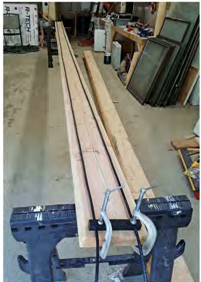
Framing lumber supported by sawhorses at each end make the construction platform.
